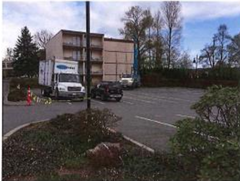
Photo 1 – Proposed building addition area looking northward. Drill rig set up at BH-1 (Photo April 11, 2016)
