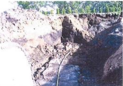
Photo 5 – Provided photo of excavation during parking lot construction in proposed building area showing random fill, buried organics and buried concrete (date unknown)
