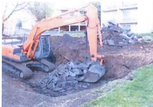
Photo 6 – Provided photo of existing parking area excavation showing buried concrete removal (date unknown)
